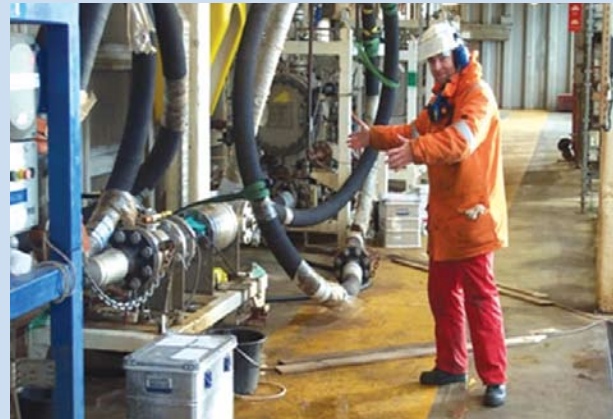
Typical North Sea CTour Test Facility Setup
